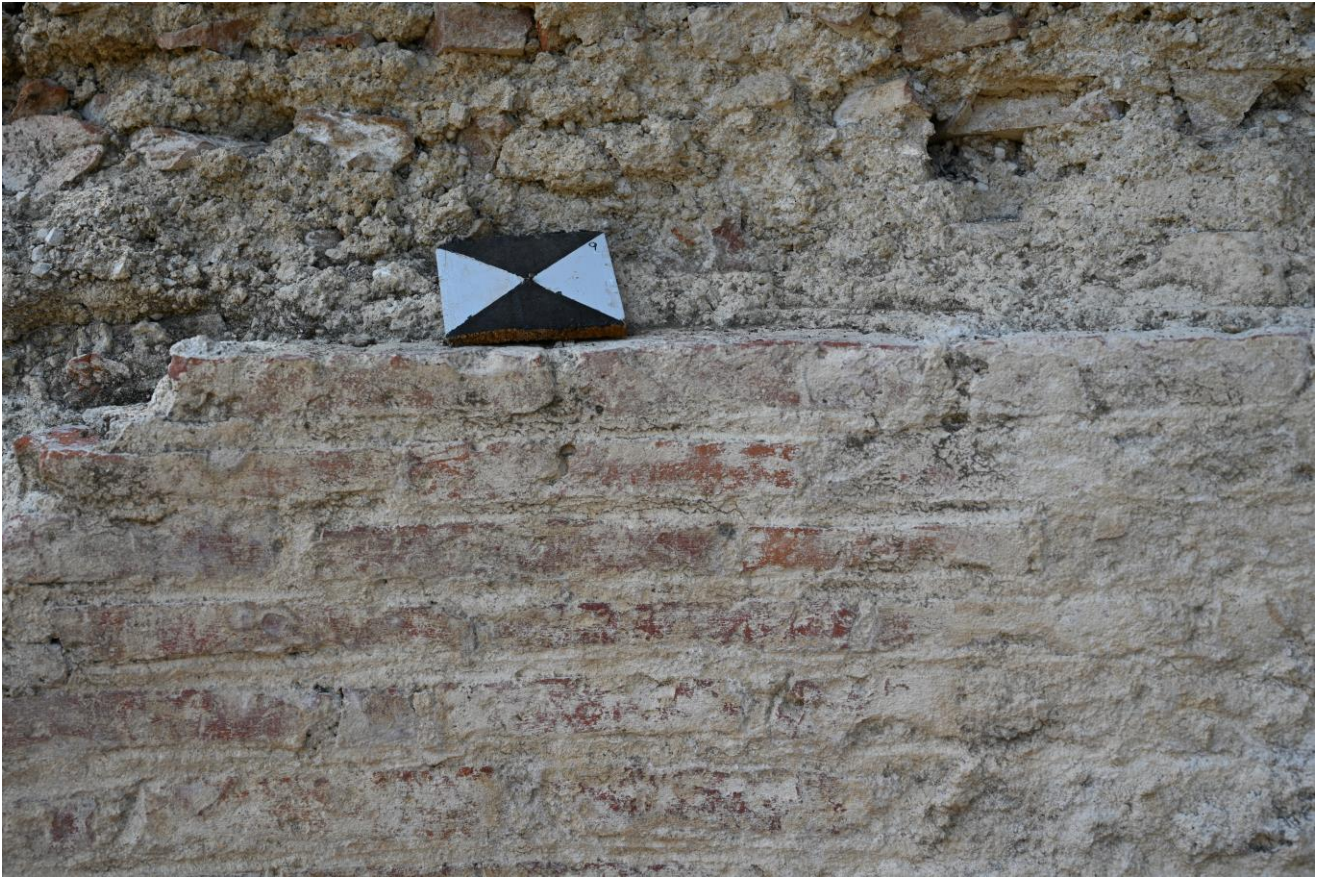
Fig. 23. Detail of opus latericium brickwork in the niche within Room 10. The drone target is 10 x 10 cm. Myles McCallum, Saint Mary's University.
