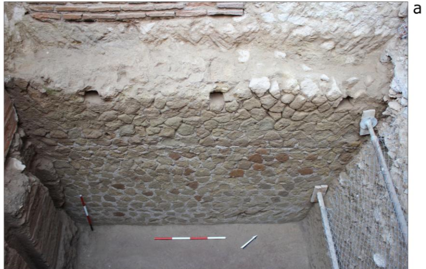
Fig. 4. a) Segment of the foundation along the back wall at southeast b) Detail of the foundations along the partition wall number 15.
