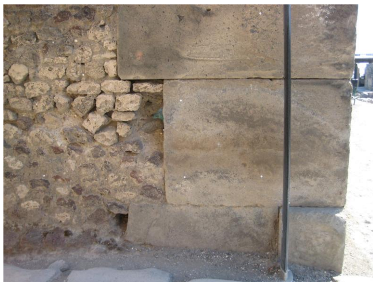
Fig. 12. Misaligned blocks in tufo nocerino on the north-east corner of Insula VII 6.
