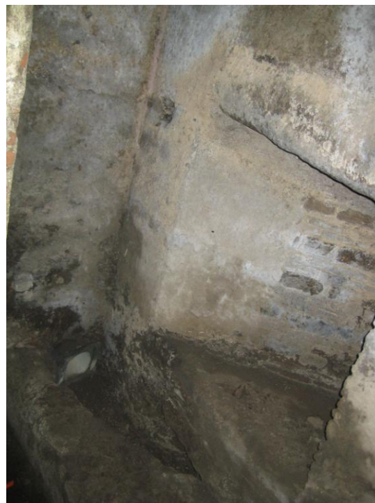
Fig. 35. Drainage with bronze fitting (lower left) and access corridor (right) within the service rooms of the 'Great Cistern.'
