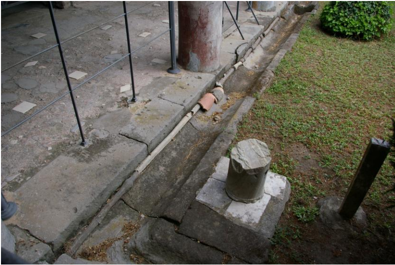
Fig. 19. House VI 16, 7.38: water pipe in Peristyle.
